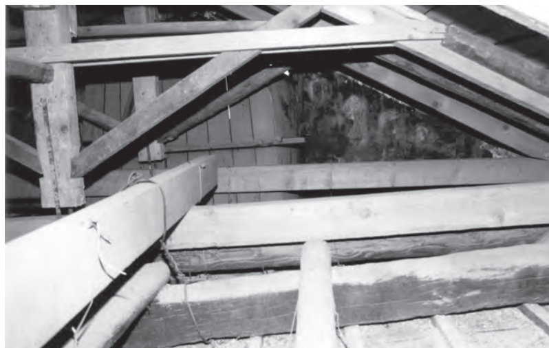
Fig. 25 Basilica of Dormition, Kalampaka, Thessaly, View inside the roof, at the back the paintings of the western wall
