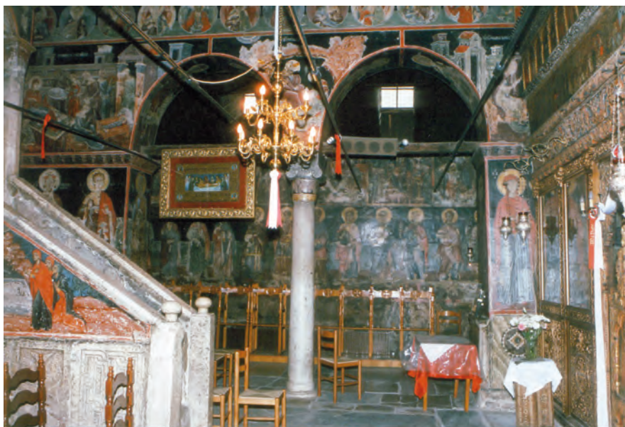
Fig. 21 Basilica of Dormition, Kalampaka, Thessaly, View of the eastern arcade of the north aisle from the nave
