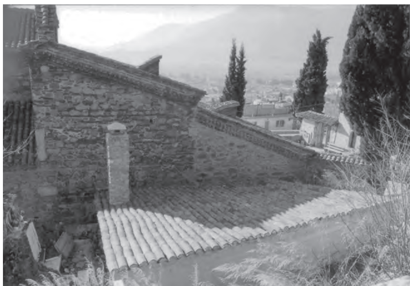
Fig. 13 Basilica of Dormition, Kalampaka, Thessaly, Western half of the north facade, with apparent construction phases
