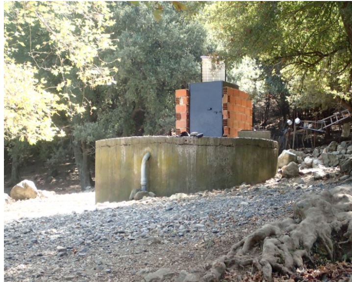
Figure 3. Cistern installed directly at a spring outflow
