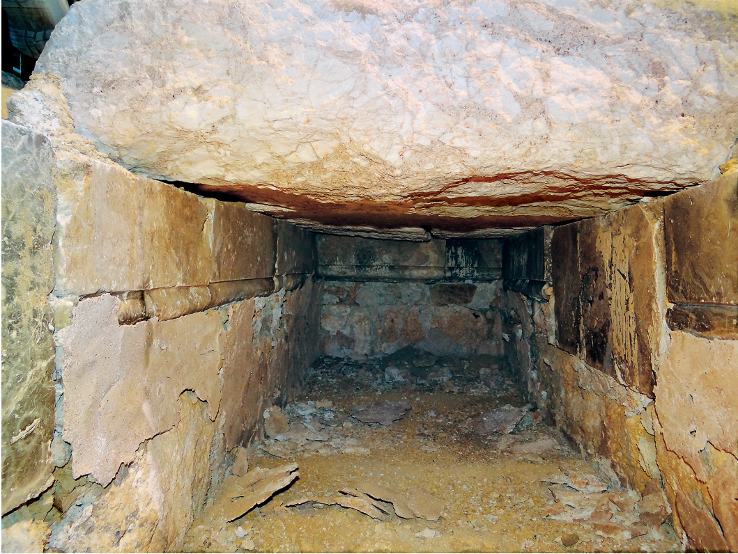
Fig. 65 Memorial of Moses. Tomb in the centre of the nave, detail of the red plaster and of the marble row.
