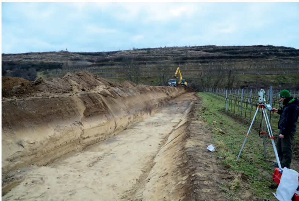
Fig. 8. Kammern-Grubgraben 2015, machine excavation to just above the cultural layer in the area of the newly planned access road (photo: T. Einwögerer, OeAI, OeAW).
